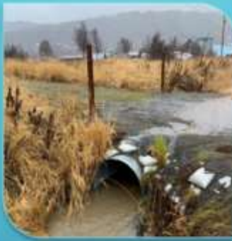
Sediment laden storm water discharges to Kachemak Bay
